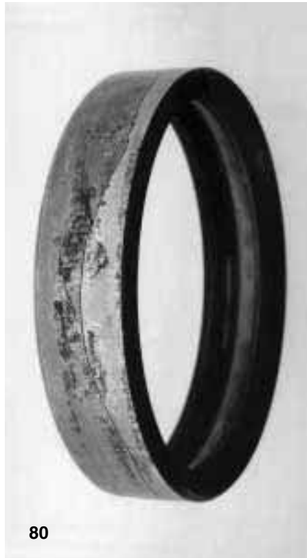
Fig 79 Spherical roller bearing inner ring with fretting corrosion and a transverse crack right through the ring. The fretting corrosion has caused the cracking
